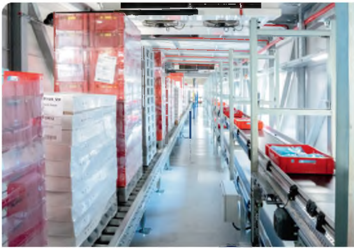
Pallets, boxes and cartons are transported automatically via a steel bridge into the new logistics centre.
